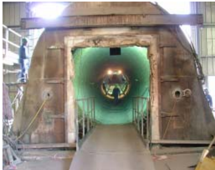
KilnGard-600SCW Application in a Cement Kiln
